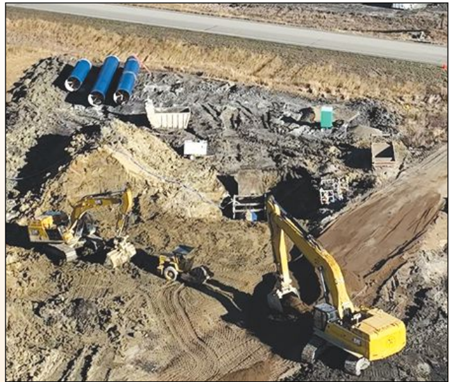
Revere Township to Cooperstown in Griggs County, including three 96-inch diameter trenchless crossings of jurisdictional wetlands. The results of the bid process will be announced in the first quarter of 2026 RRVWSP newsletter.
